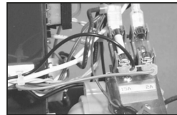
Figure N - Fuses
